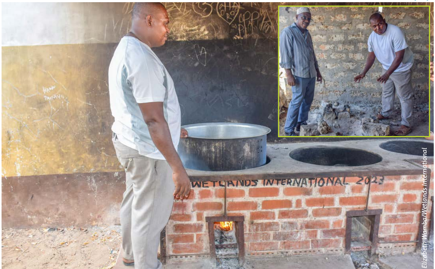
A commercial improved cookstove at Pate Primary School, serving 800 pupils and staff. Inset: the old three-stone stove
